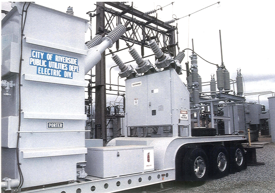
MVA Mobile Substation
