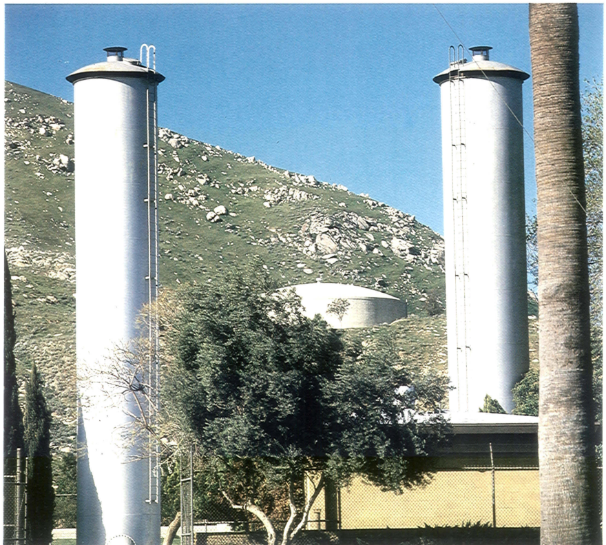
Pipeline booster station with surge towers and a reservoir in the background.
